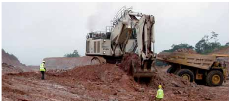
Mining slope with geological staff supervising the select mining activities of a 295 ton excavator
