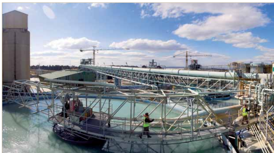
1 Processing Plant, Driefontein
